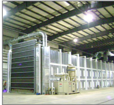
Large equipment enclosure, electric rubber doors
